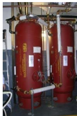
Figure 3 DHW STORAGE TANKS
